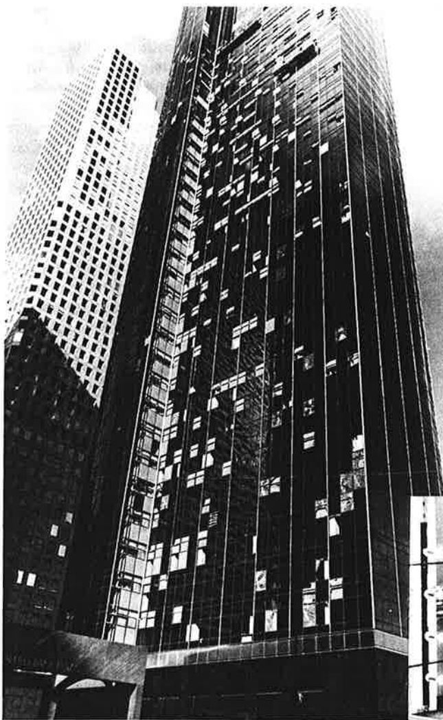
Houston buildings after Hurricane Alicia. Note window glass broken by wind pressure and windborne debris from the August 1983 hurricane.
